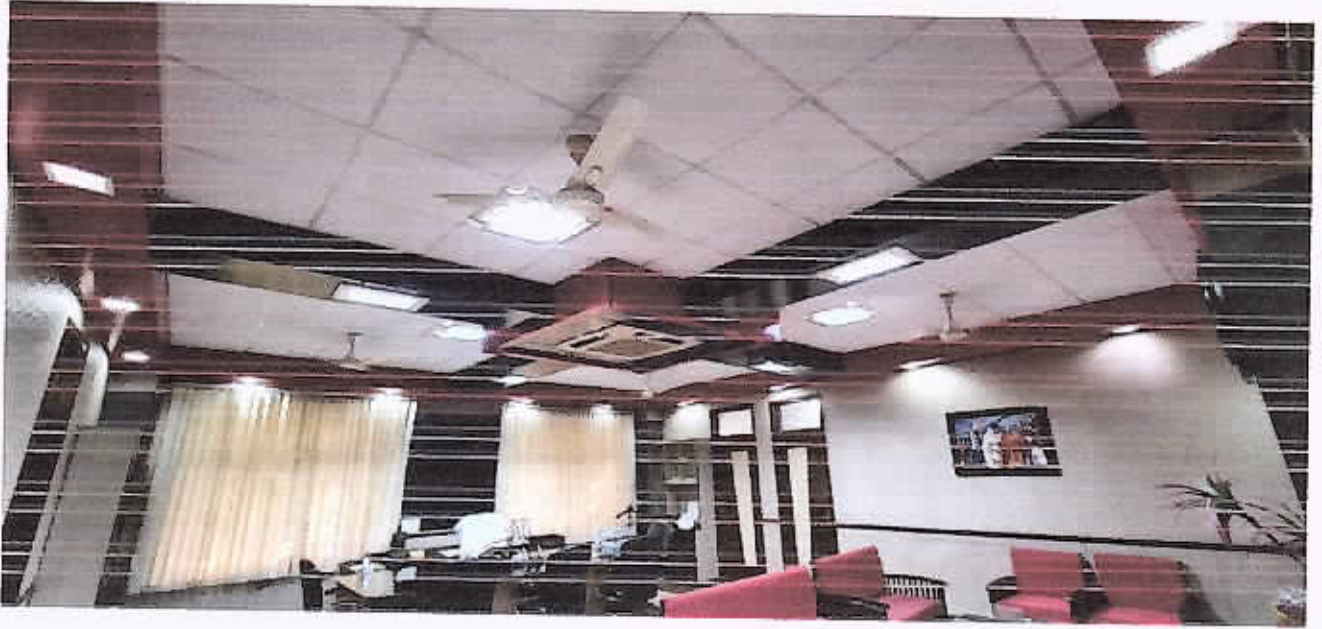
LED Ceiling Lights in Office
