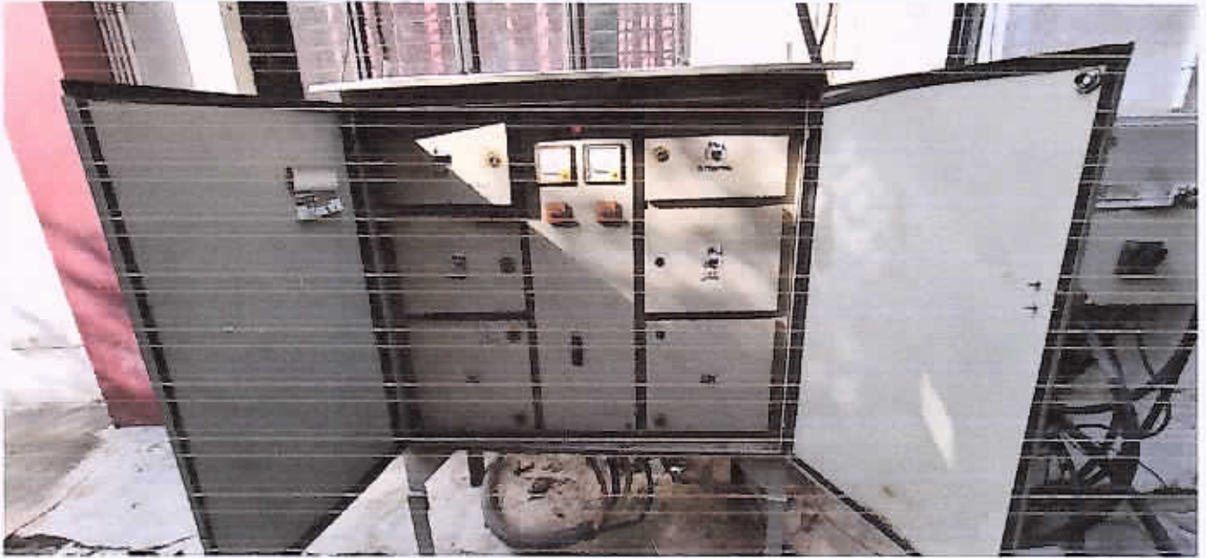
Electric Sub-Station in Block-3
