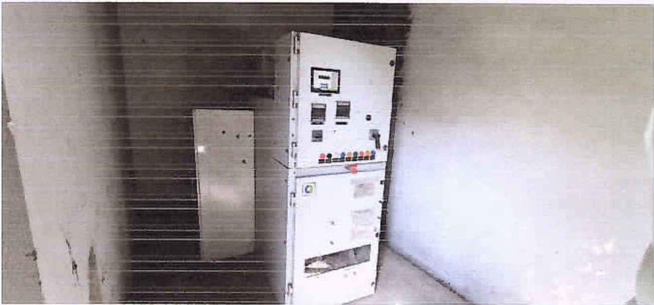
HT Breaker in Sub-Station
