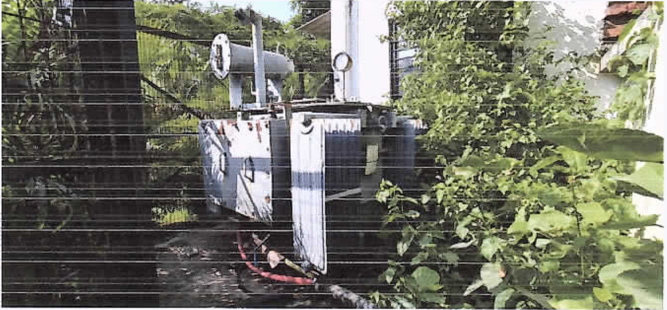
Transformer at Sub-Station
