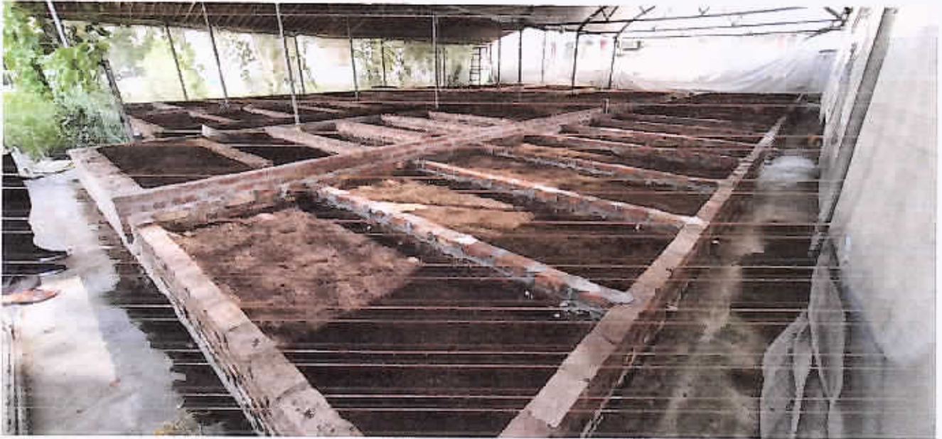
Bio Gas Plant
