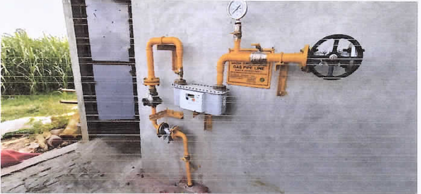
LPG Station in Hostel
