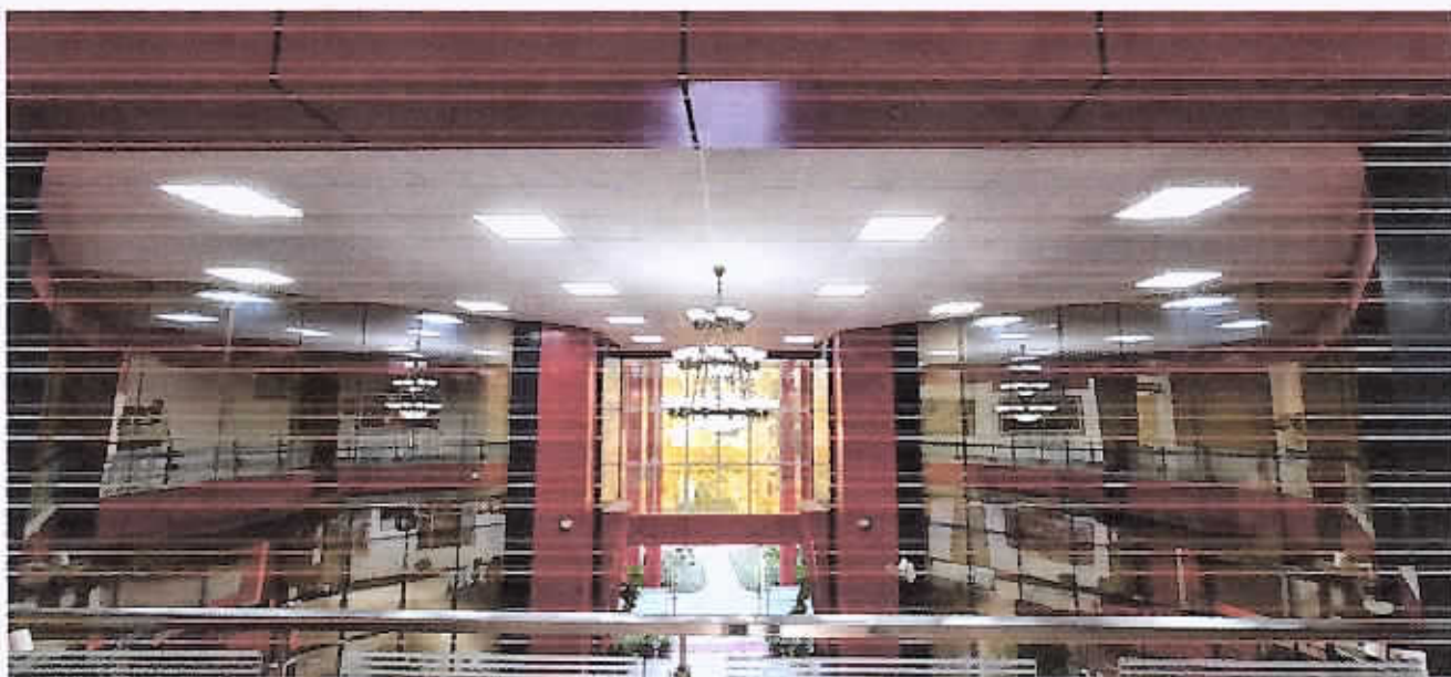
LED Ceiling Lights in Lobby
