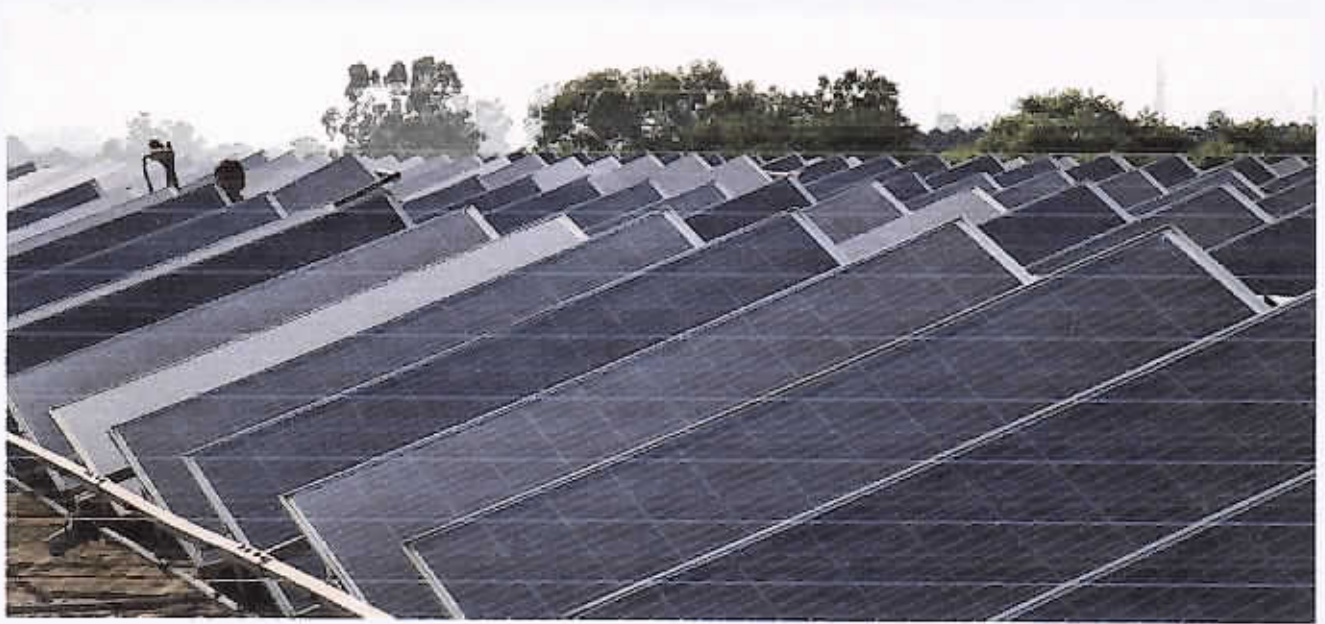
Solar Panels on Roofs
