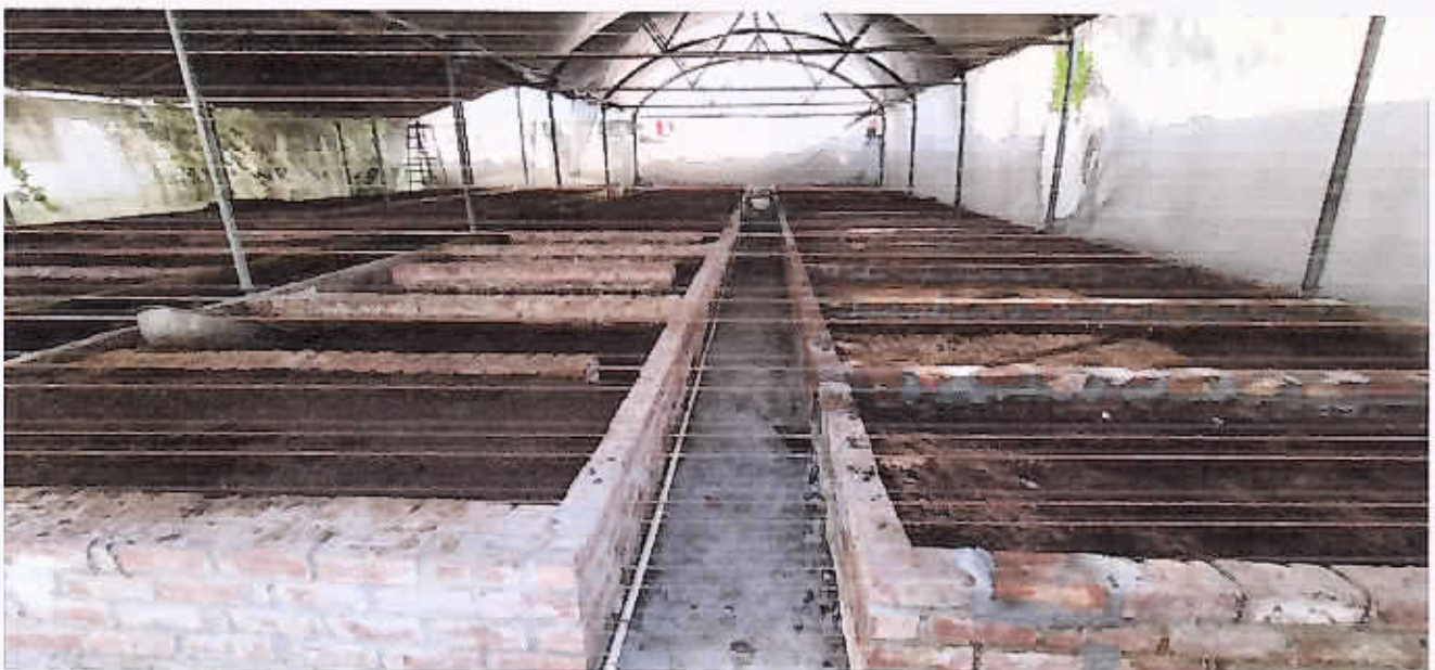
Bio Gas Plant
