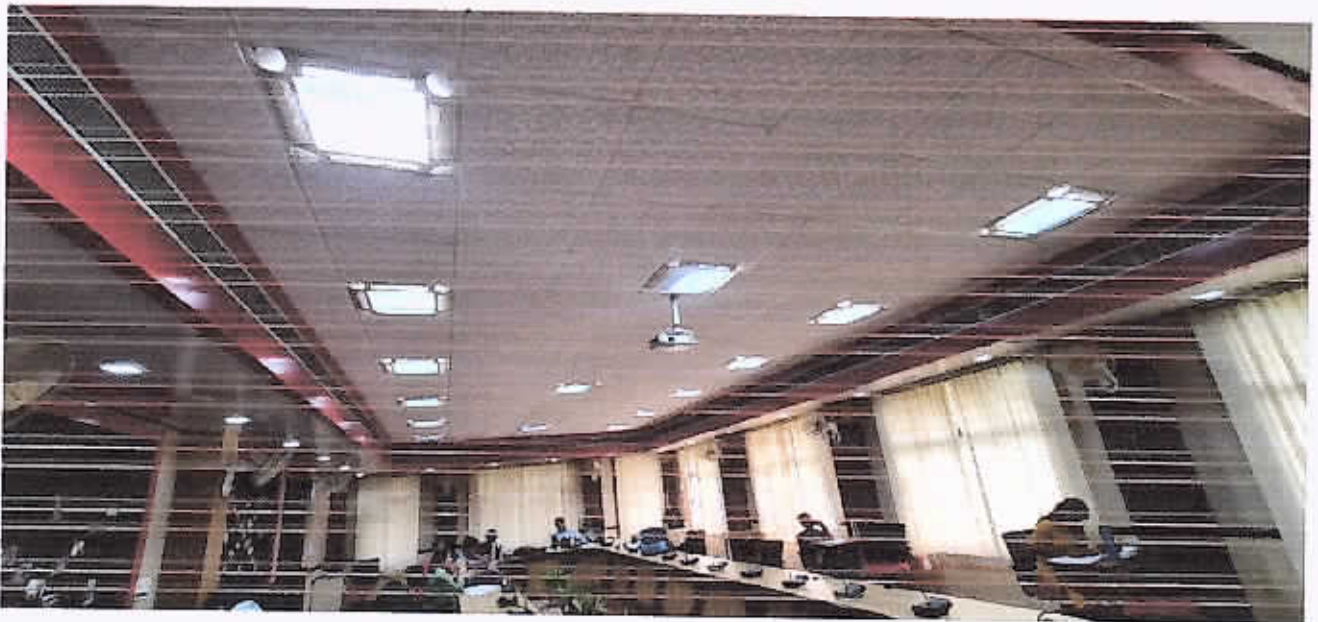
LED Ceiling Lights in Conference Hall
