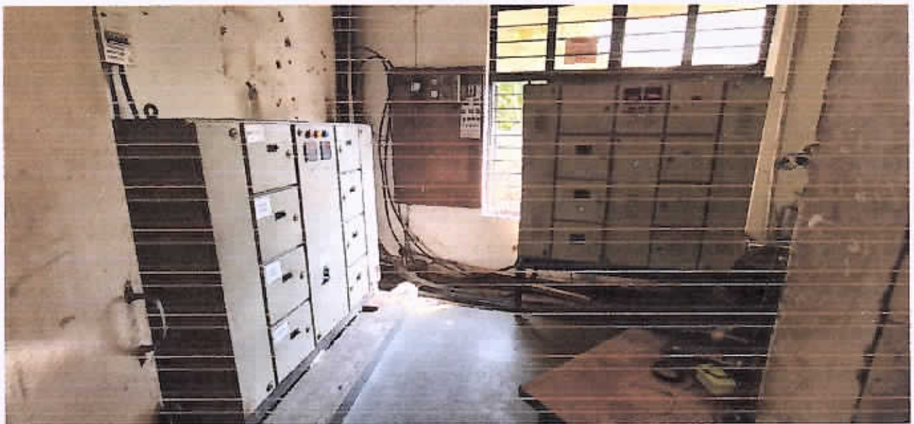
Electric Sub-Station in Block-2
